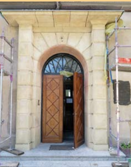
14. Prace restauratorskie przy kamiennym portalu dawnego Biura Budowy Portu 14. Restoration works at the stone portal of the former Port Construction Office
