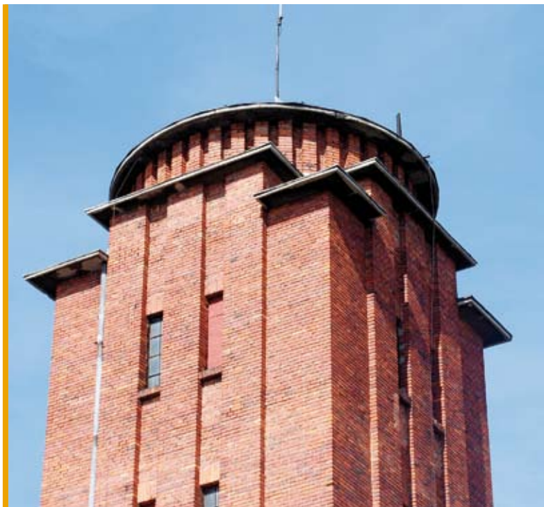
8. Toruń, new municipal gasworks, tower of the apparatus building, Lubicka 52-58 street, 1938-1942, (photo Jakub Polak, 2017)
